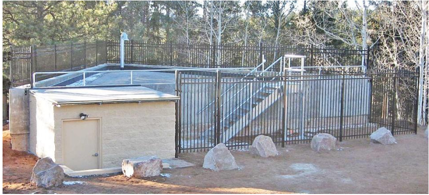
Our Renovated 75,724 Gallon Tank & Plumbing Vault
